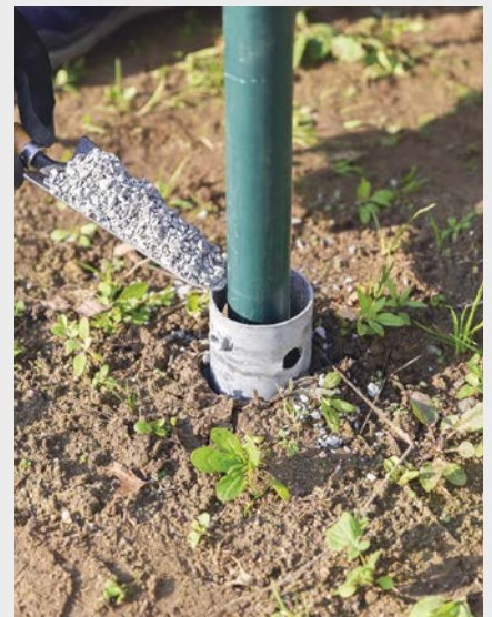
6 Set the post in the support by back-filling it with granite grit, so that it is stiffened and locked in place.
