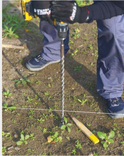
2 Using a long drill bit, drill a pilot hole to check the ground and remove minor obstructions.
