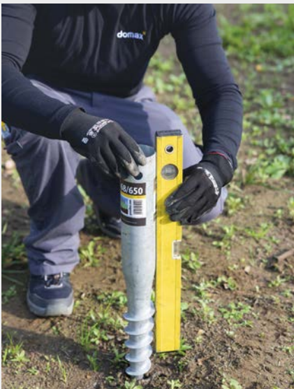
4 Use a spirit level to check the correct alignment of the post supports.
